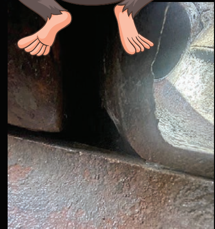
Intersecting pipes and ducts create voids which installers often neglect to fill.
