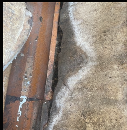
Benching often deteriorates after long exposure to splashing water.
